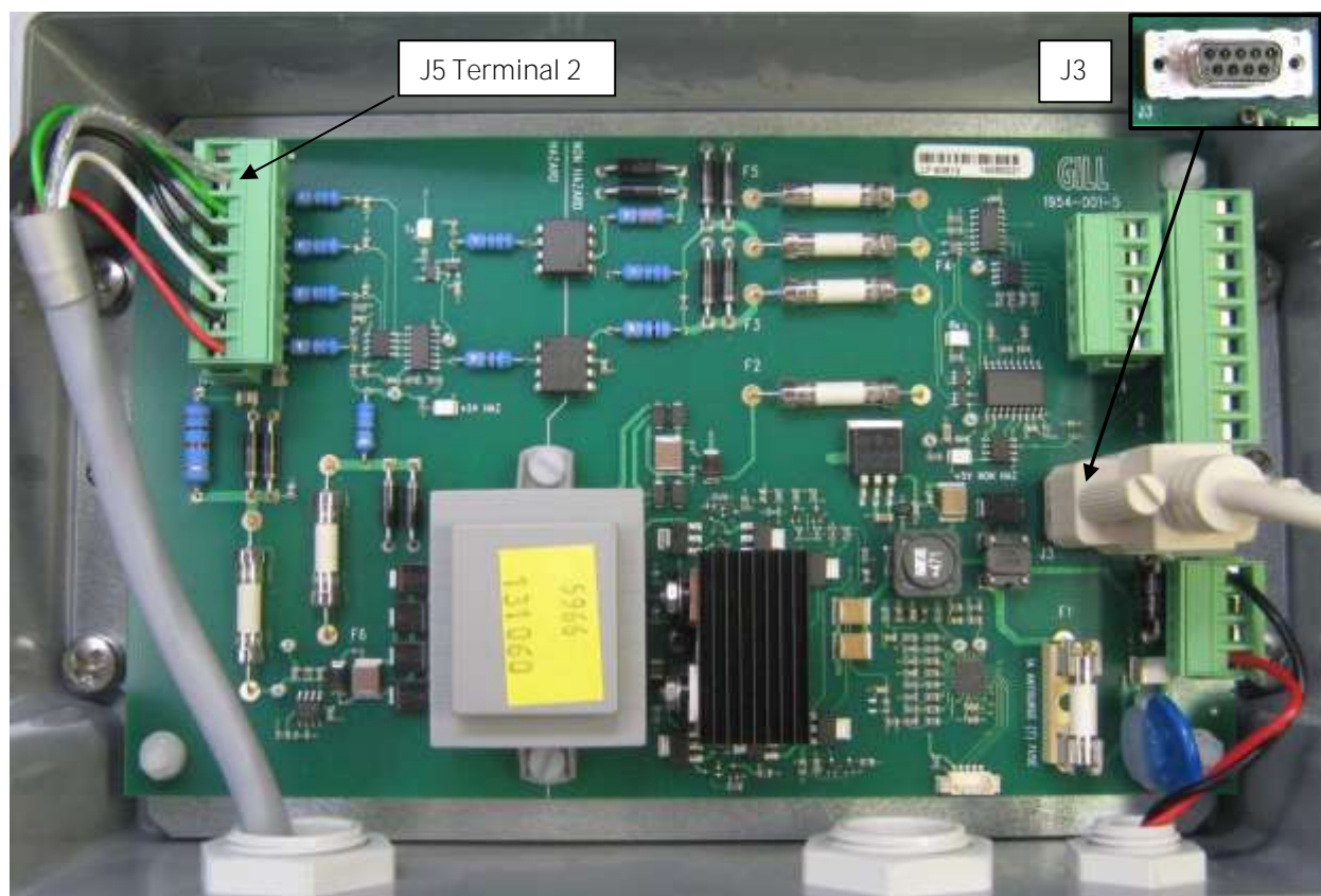
IS WindObserver 3 Metre Test Cable Connection Table to LVPCI Box J5.
